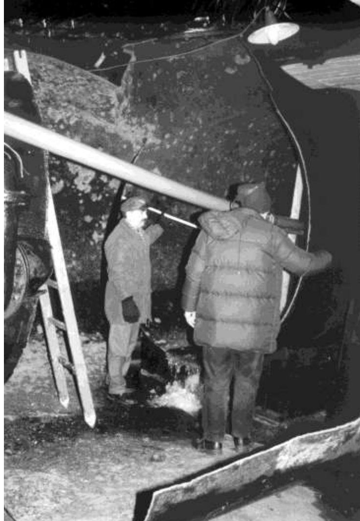
Disrupted penstock in the Łapino Hydropower Plant
