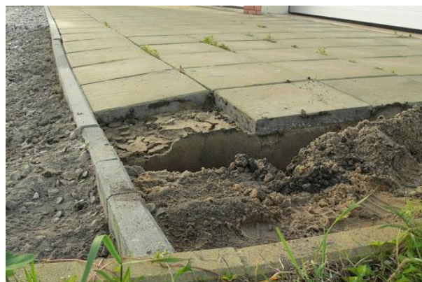
Fig. 1. Visual effect of collapsing pavement structure due to unstable subsurface
